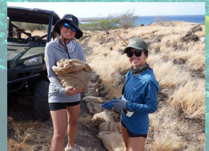
▲ Volunteers Naomi and Peyton Tokishi working on roadway repairs to reduce sedimentation
