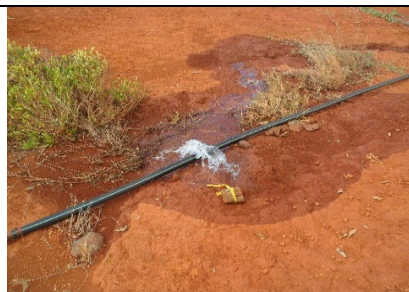
A blow out on a 1.5 inch irrigation main
